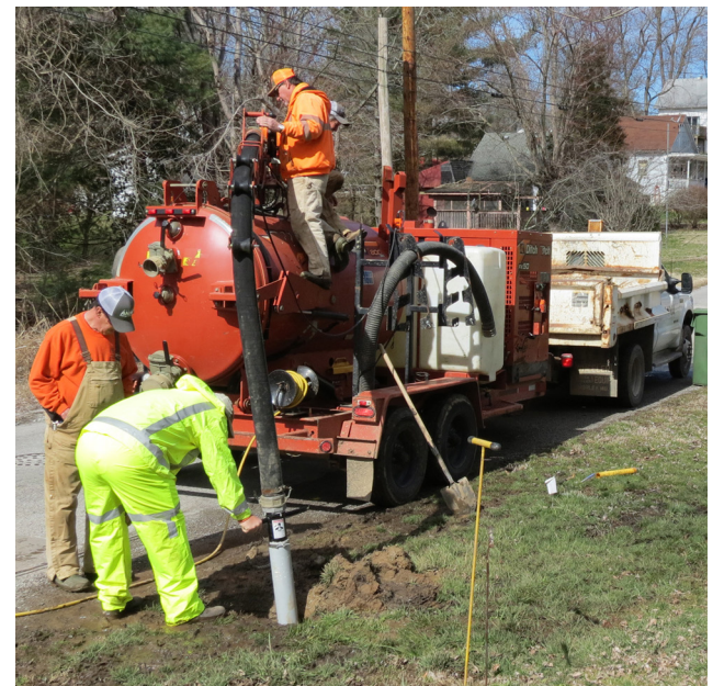
Hydro vac at work: The city recently acquired a hydro vac which was utilized for a water line repair project. The equipment uses high-pressure water for removal of dirt.
