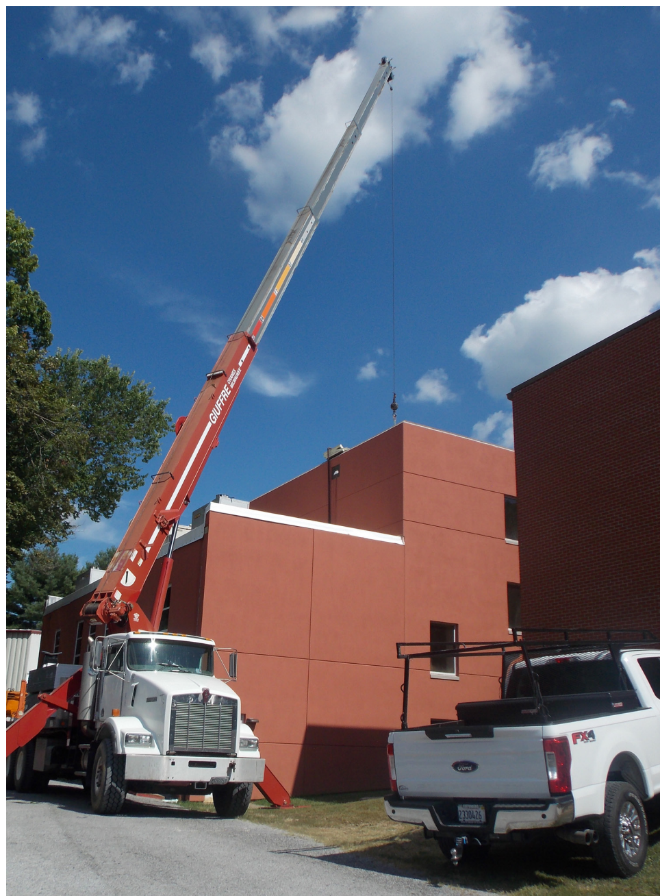
Anna School District Cranes moved material to the top of Anna Junior High School as part of a summer construction project for Anna School District 37. Roof construction has been scheduled for the oldest parts of Anna School District buildings, including both cafeterias and the band room. Photos by Benjamin Marxer.
