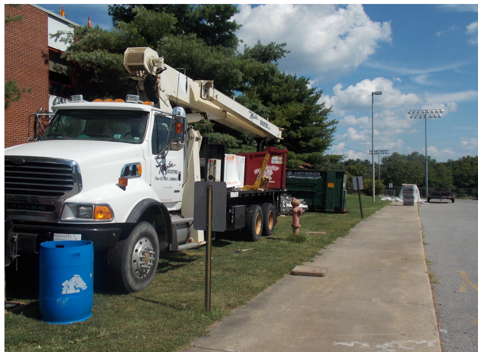
Anna-Jonesboro Community High School Repairs and upgrades are underway this summer on the roof at Anna-Jonesboro Community High School. Paving and sealing work also was slated at the school.
